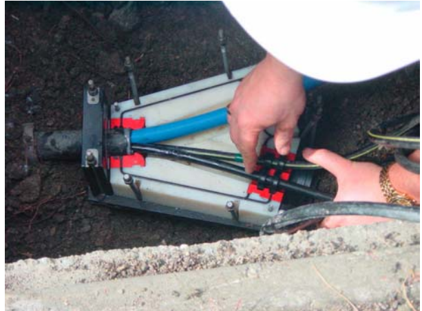
Figure 7. Mounting Y-piece for additional jetting with 2 resident cables and guide for the tube
