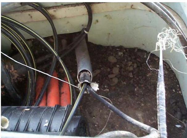
Figure 6. Duct occupied with 2 resident cables
